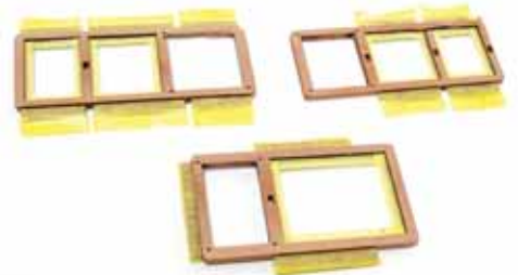
258. Mask the cannon ball garlands and the openings that will be fitted with a grating. Keep the stairway openings unmasked. Paint the assemblies in black.
